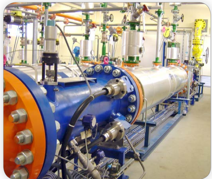
Gas Verbund Mittelland (GVM) natural gas pressure let down recovery station can deliver a total of 600 kW (2 stages).
